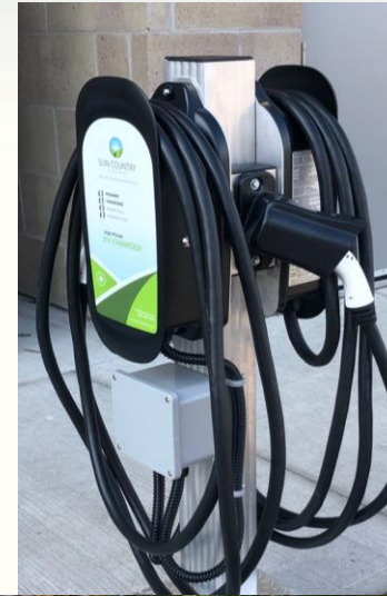
Photo: Collingwood Redevelopment EV charging station
