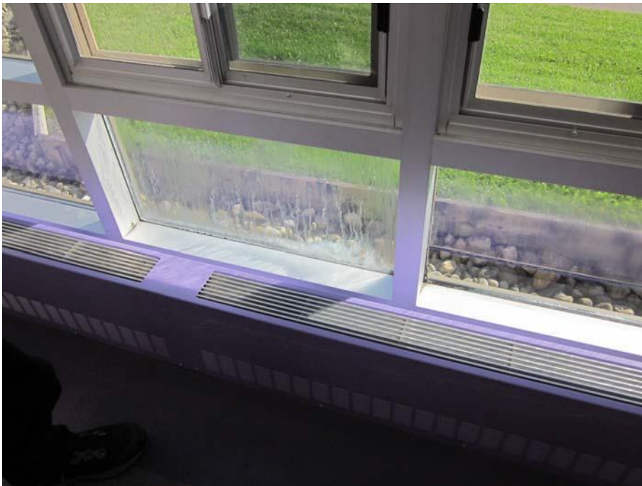
Image 2: Building Envelope – Failed Glazing Unit
