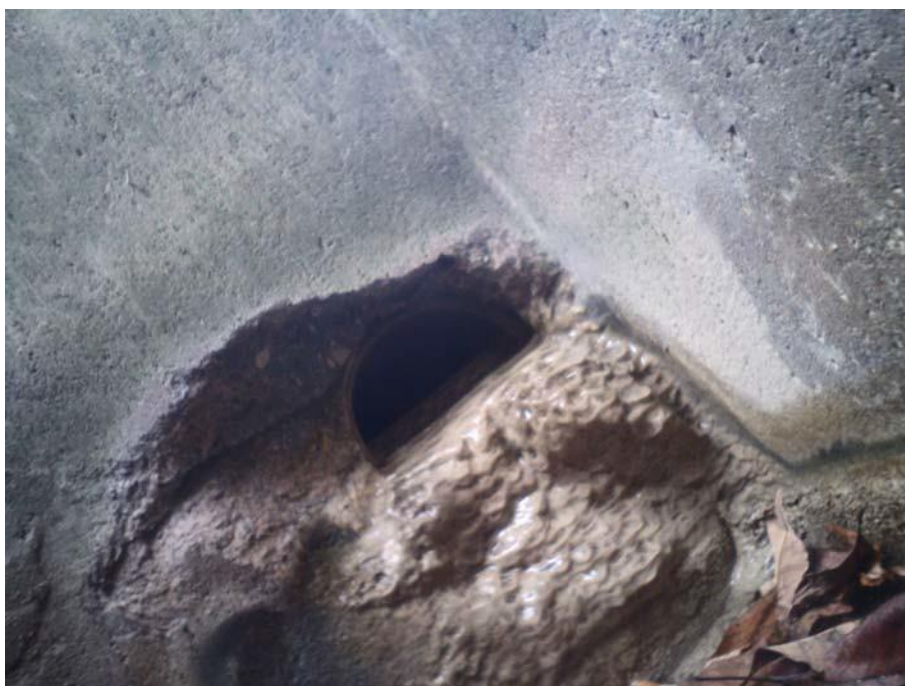
Image 7: Site Conditions Calcified Drain Lines
