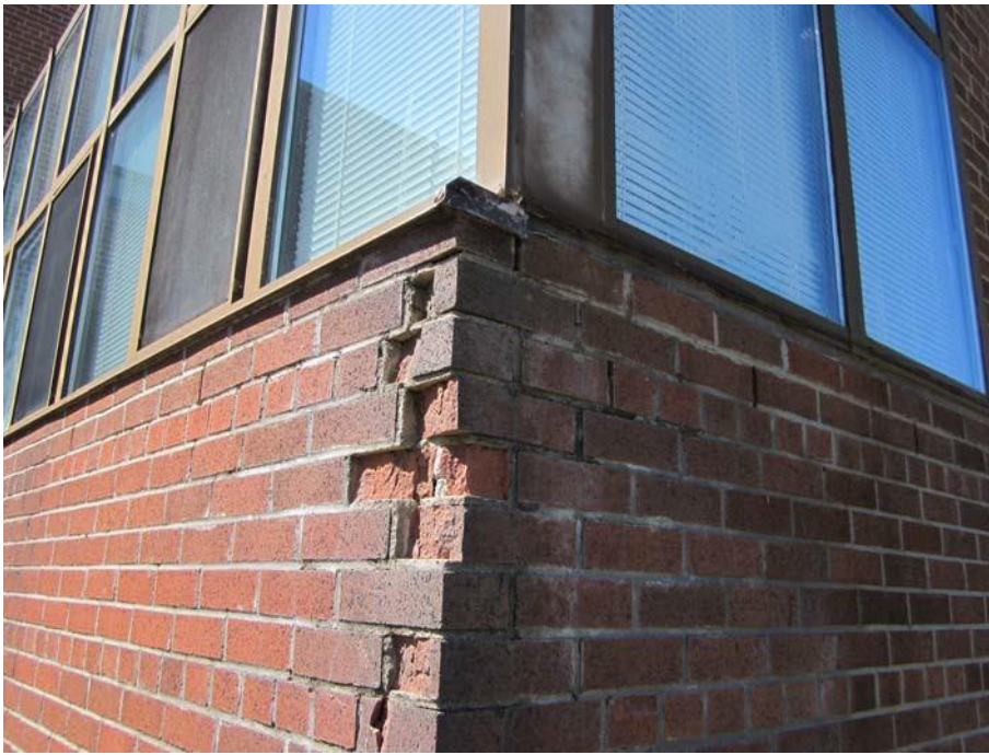
Image 1: Building Envelope – Brick Cladding Failure
