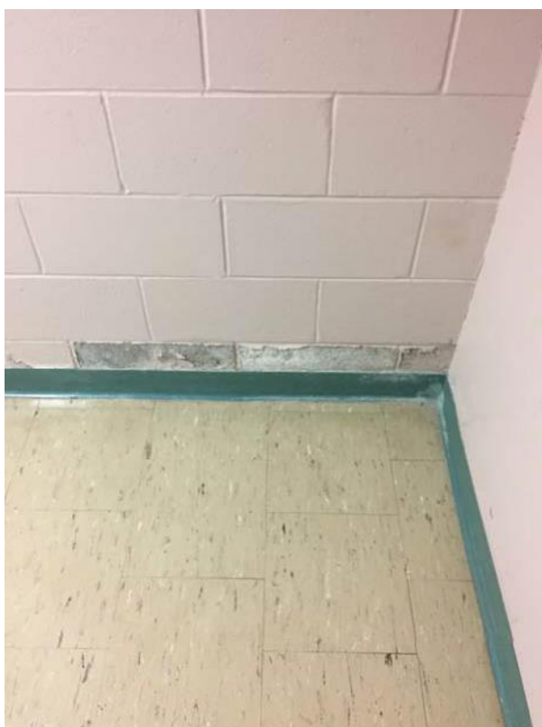
Image 8: Interior Conditions – Water Damage
