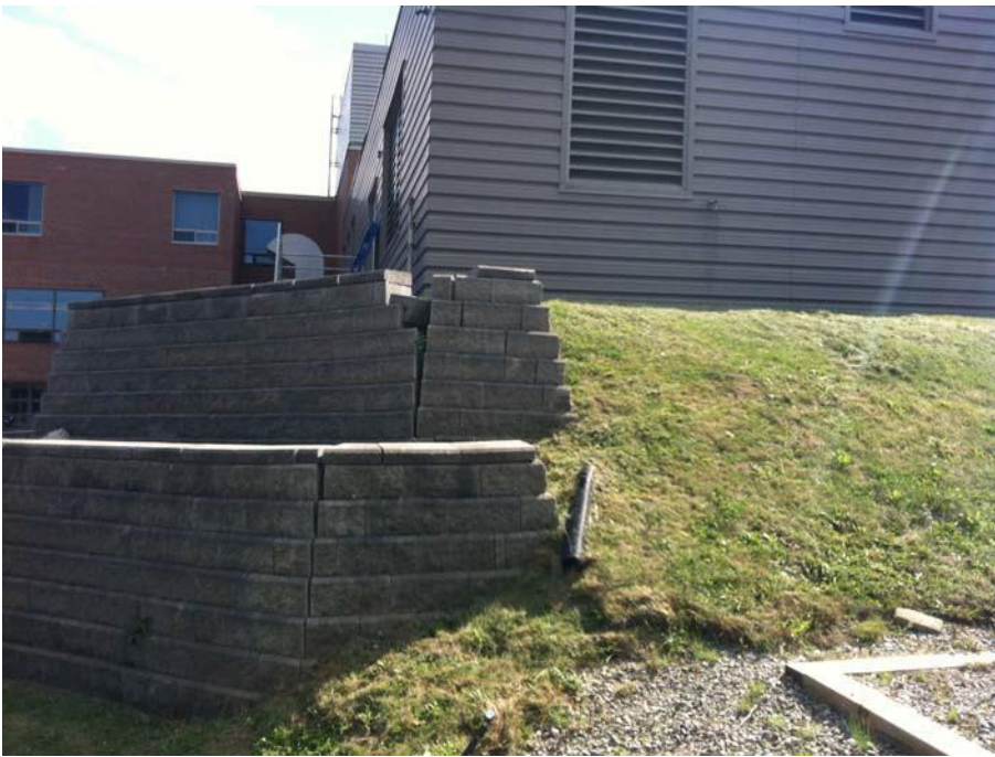
Image 3: Existing Site Condition – Failing Retaining Wall
