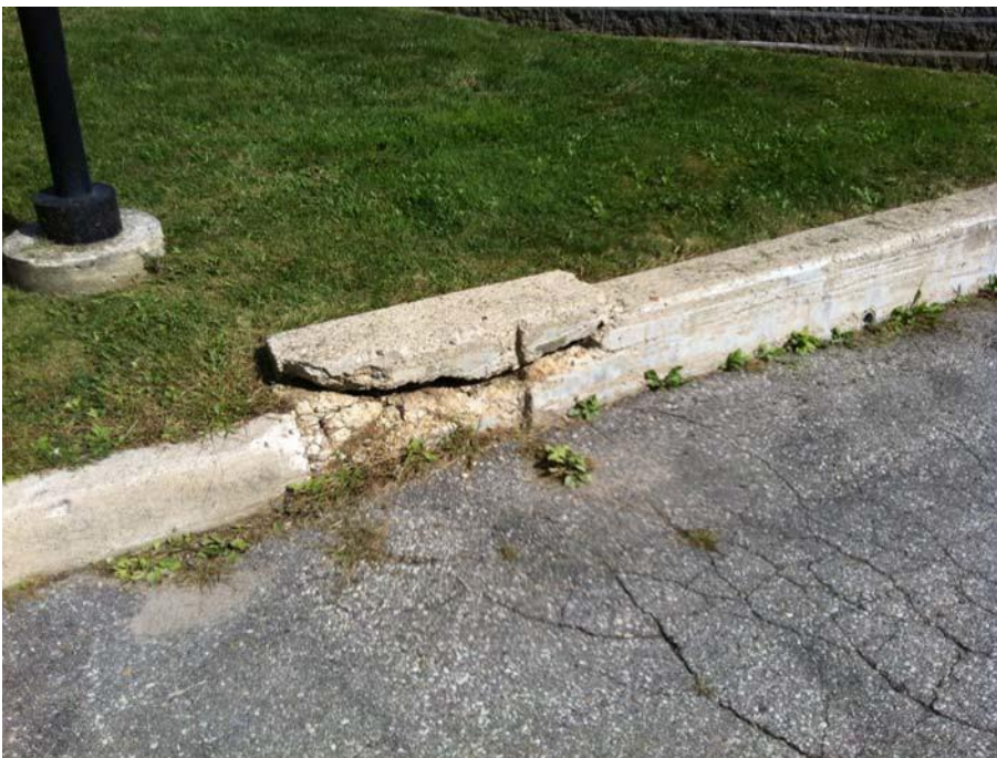
Image 4: Existing Site Condition – Broken Asphalt Paving and Curb
