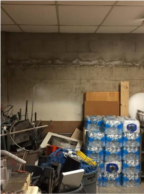
Image 9: Interior Conditions – Water Damage
