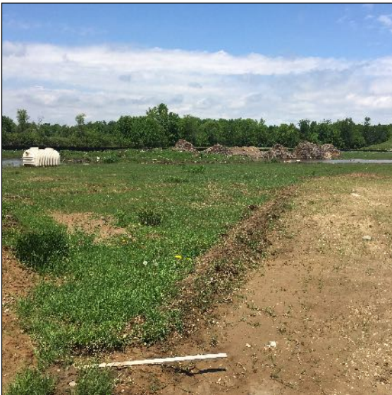
Image 7: Disturbed soil conditions showing grading.
