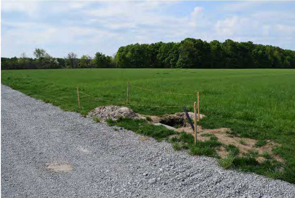
Image 5: Field conditions at TL3, note grass colour variation along edge of road indicating buried conduits, facing southwest.
