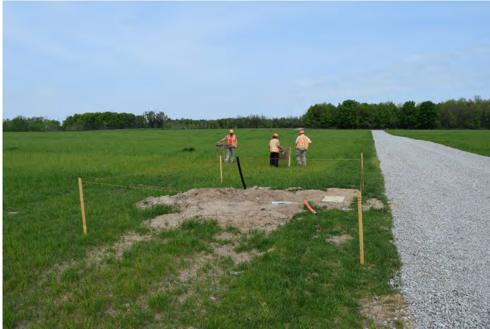
Image 1: Test Pitting at TL1, note grass colour along road edge from installation of conduits, facing northwest.
