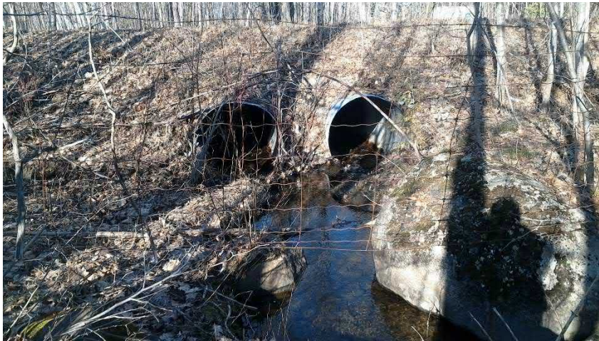
Photo 1. Twin CSP culverts which convey the intermittent watercourse eastward beneath Carriage Court (24 April 2019).
