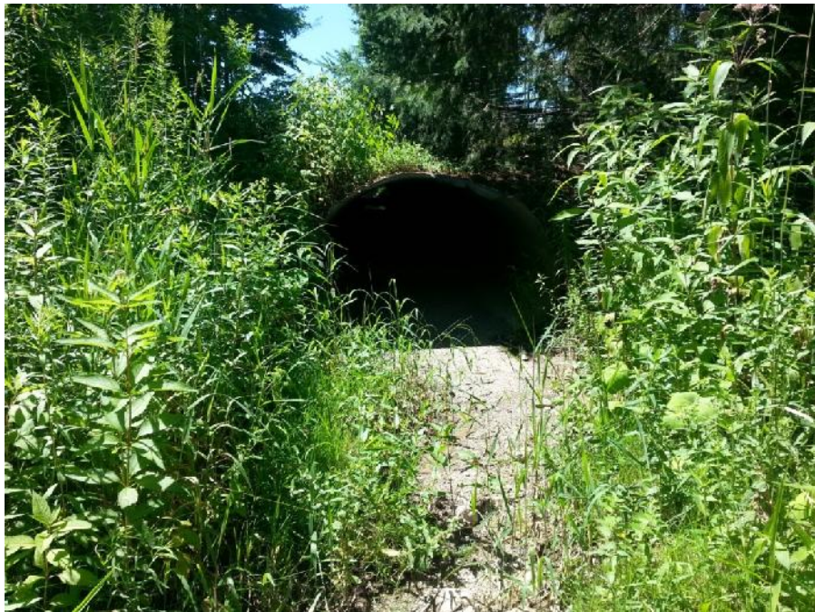
Photo 42. Burl's Creek. Photo of downstream face of Culvert 4. Located approximately 448 m from the northern property boundary.
