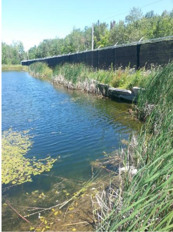
Photo 1. SWM Pond 1. From south facing north east showing unstable engineered concrete bank.
