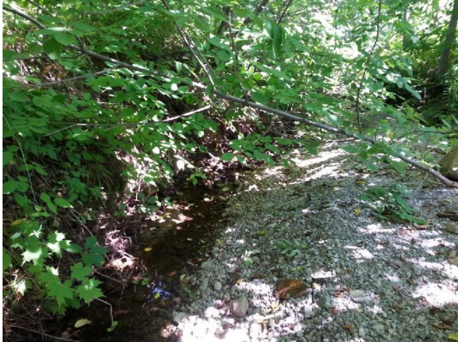
Photo 25. Burl's Creek, photo facing downstream from Culvert 2. Excess gravel noted in this area.
