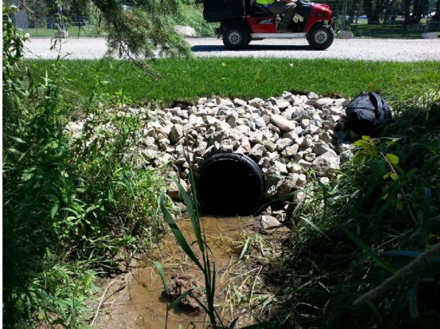
Photo 37. Burl's Creek, photo of upstream face of Culvert 3 located approximately 341 m from northern property boundary.
