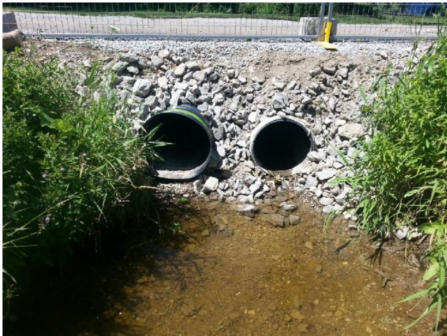
Photo 38. Burl's Creek, photo of downstream face of twin Culverts 3a and 3b, located approximately 348 m from the northern property boundary.
