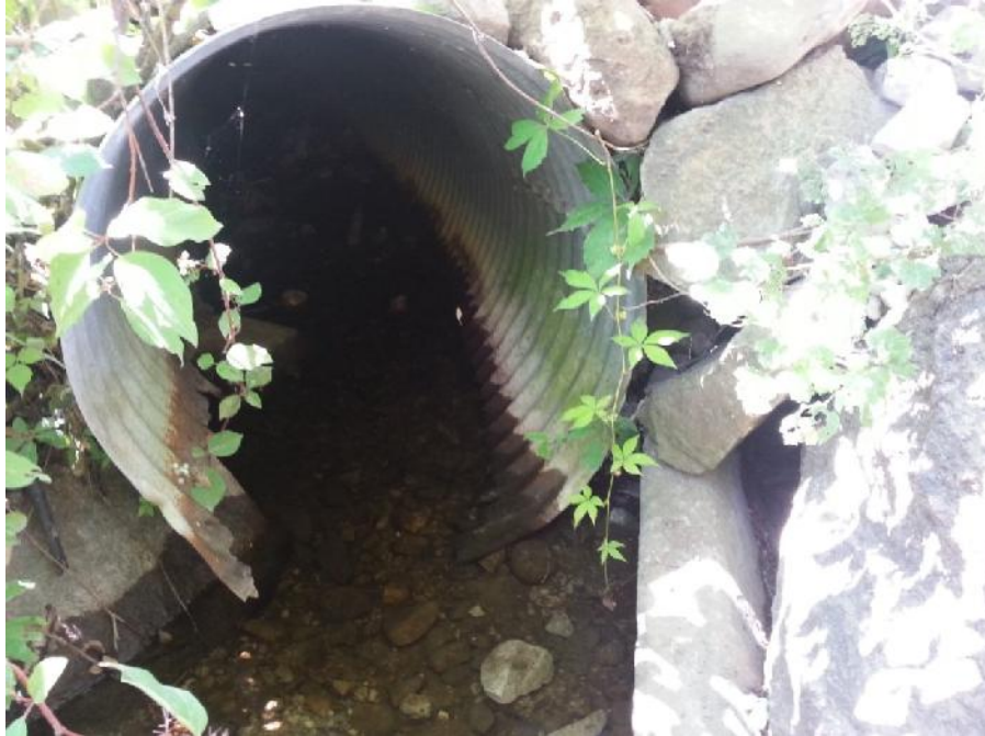
Photo 23. Burl's Creek, photo of upstream face of Culvert 2. Photo from upstream (north) facing downstream (south).
