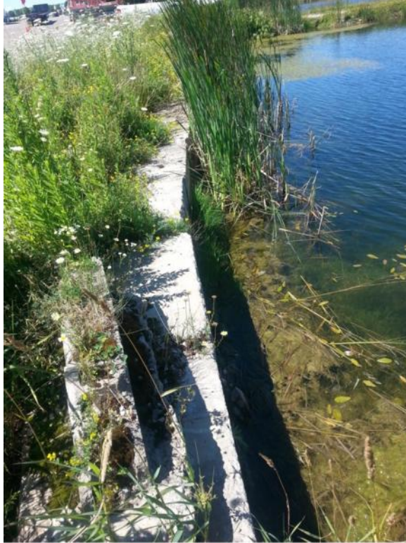
Photo 3. SWM Pond 1. Close up of south bank showing engineered concrete block bank and algae bloom.
