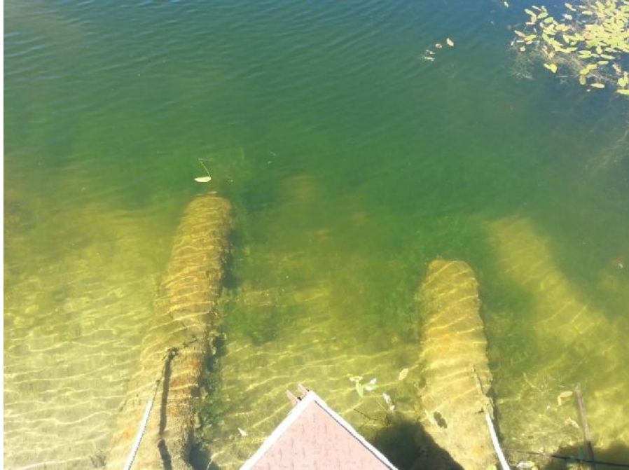
Photo 9. SWM Pond 2, north arm. Close up of twin culvert outlet to 8th Line.
