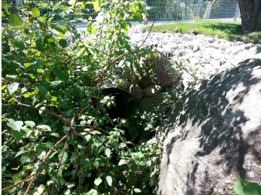
Photo 21. Burl's Creek, photo of downstream face of Culvert 1. Photo from south looking northwest at the property boundary (fence in background). No photo of upstream face of culvert 1 as it is outside of property boundaries.
