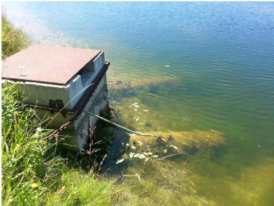
Photo 8. SWM Pond 2, north arm. Photo of twin culvert outlet to 8th Line.
