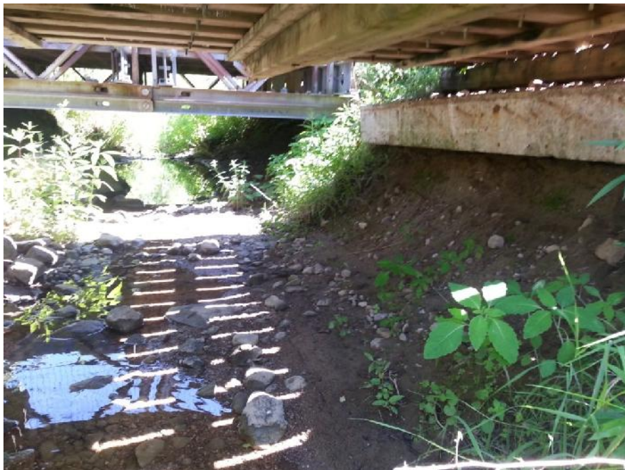
Photo 36. Burl's Creek, photo of right bank of Bridge 4 located approximately 265 m from northern property boundary.
