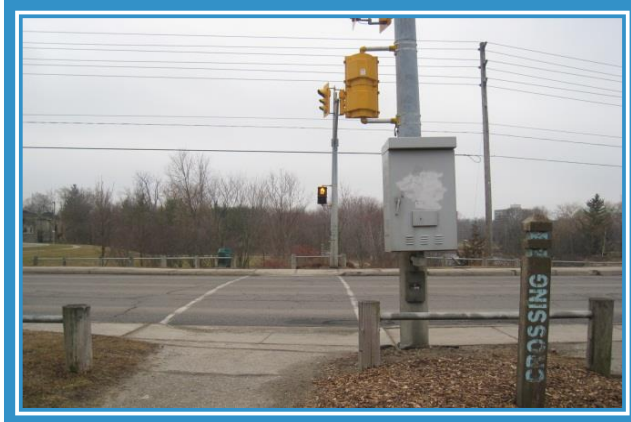
Midblock Pedestrian Signal Without Median Credit: MMM Group, 2012
