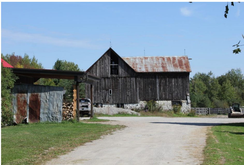
Agricultural Facility # 21 – bank barn (missing wall boards), residential unit, shed
