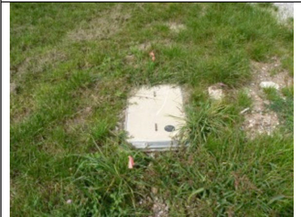
IMAGE 47 DISTURBED – SHOWS ELECTRICAL INFRASTRUCTURE
