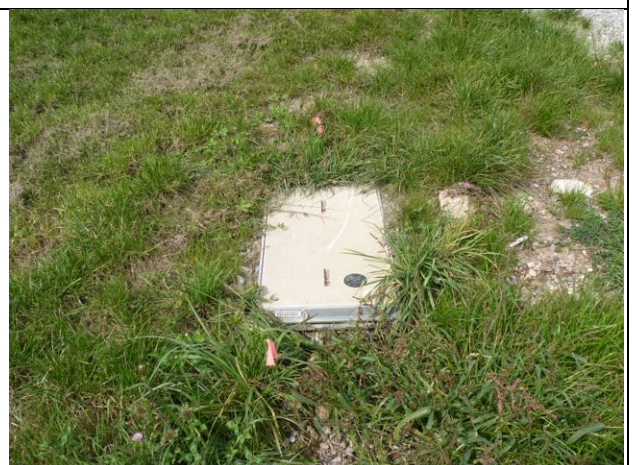
IMAGE 47 DISTURBED – SHOWS ELECTRICAL INFRASTRUCTURE
