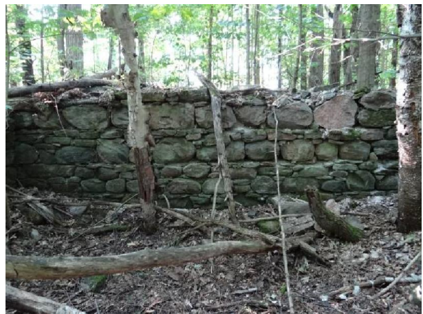
Plate 8: Interior view of south foundation wall, note the design of the alternating stone courses.
