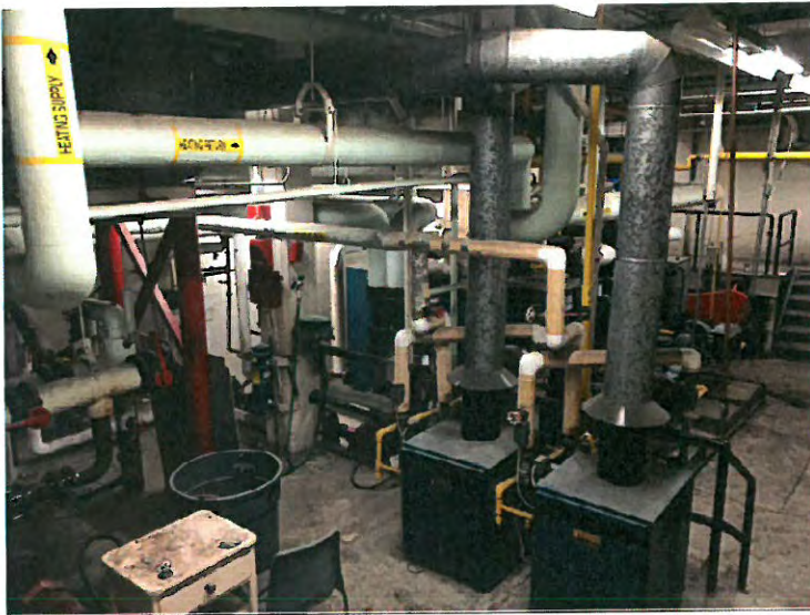
PHOTOGRAPH 4: Boiler room inside building.
