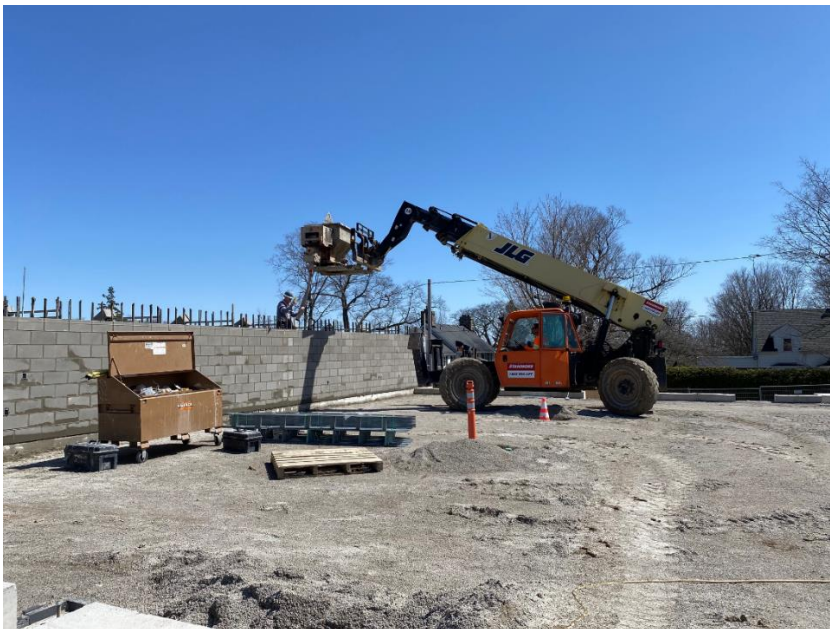
Mason grouting half the constructed wall. This wall dissects the childcare area and EarlyON
