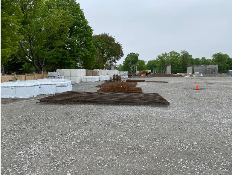
Relocation of rebar onto parking lot and view of all the roofing materials.
