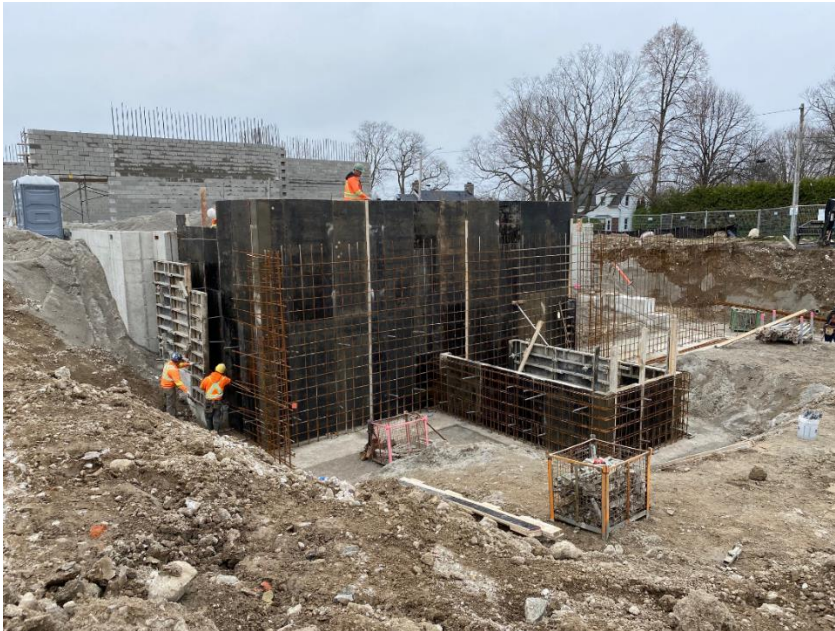
Wall and elevator pit back forming complete so waterstop and rebar inspections can take place.
