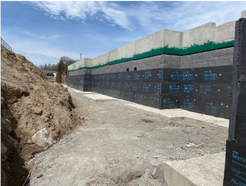
Insulation installed on exterior walls. Ready for weeping tile to be installed and then backfilling can commence.
