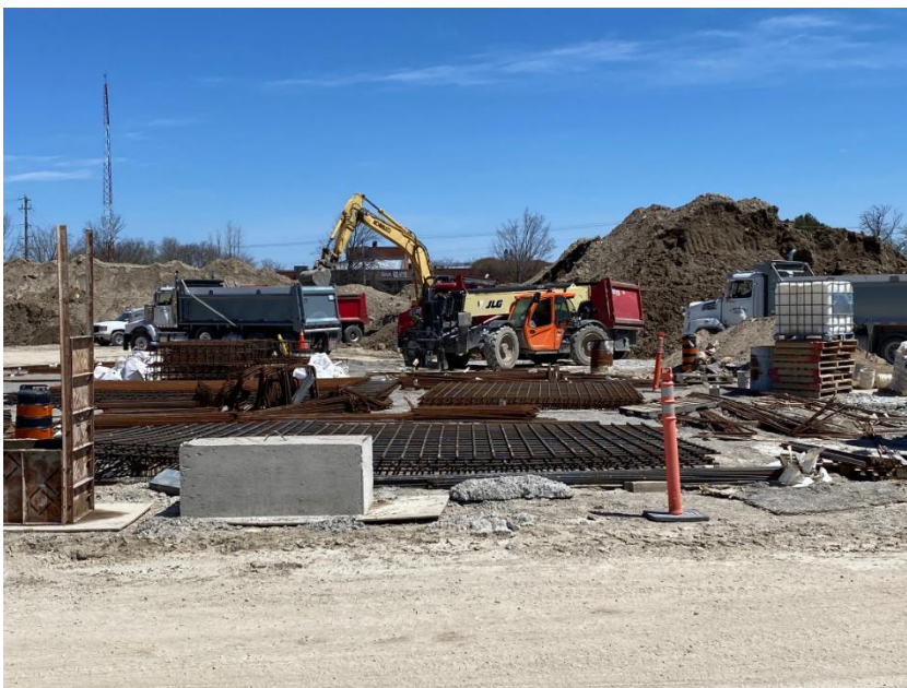
Half loads have been lifted so we are now starting to remove excess soils from the site.
