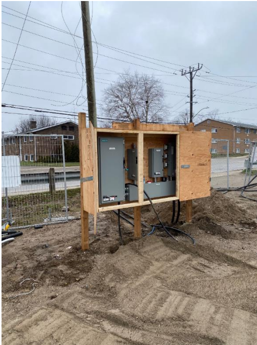
Temporary power enclosure completed. Hydro One to hook up to grid shortly.
