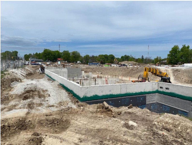
Start of backfilling the excavation around the foundation with fill from the stockpile.
