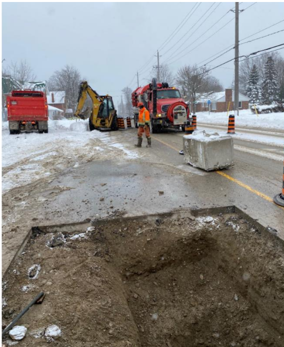
Domestic cold-water feed brought onto the property – Great teamwork with the City of Orillia
