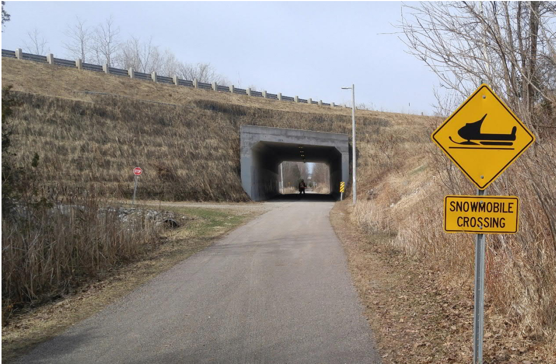
Photo 7: General view of the tunnel structure to the east of Old Fort Overhead Bridge
