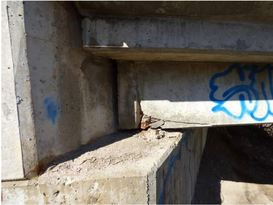
Photo 3: Bearing cracks at ends of girders (Note: picture obtained from 2016 Biennial Inspection Report by Engineered Management Systems Inc.)
