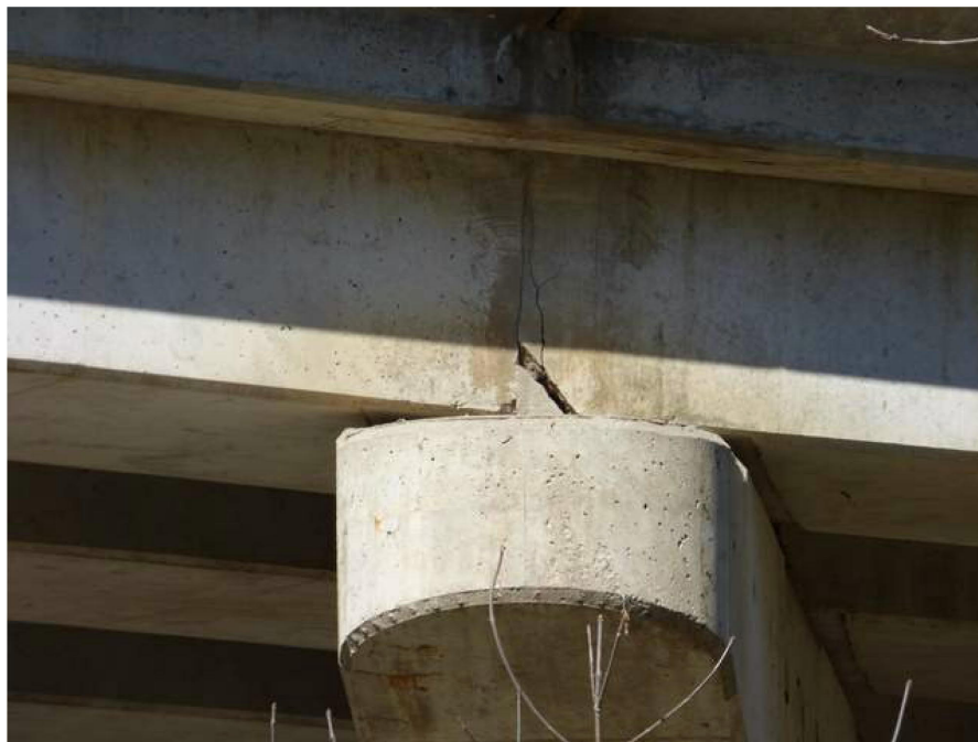
Photo 4: Bearing cracks of girders over piers (Note: picture obtained from 2016 Biennial Inspection Report by Engineered Management Systems Inc.)
